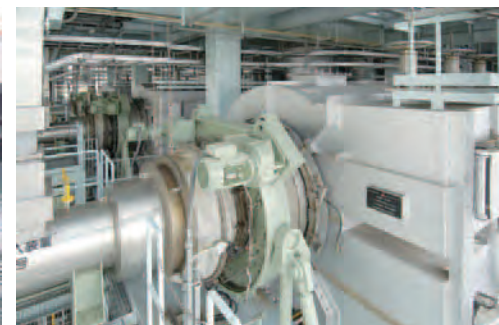
废弃物用焚烧炉 Incinerator for Waste
